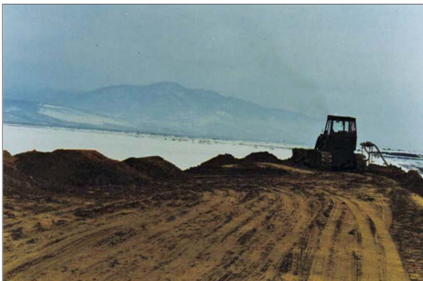
Figure 4: The breached dam of the Aurul tailings pond with machines compacting the new dam (mokka.hu, etk.hu)
